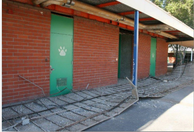
Damage to Jefferson Elementary School, Calexico, CA in the aftermath of a 7.2 magnitude earthquake in April of 2010.
